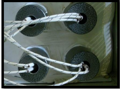
Electric Heater (Behind the lower door)
